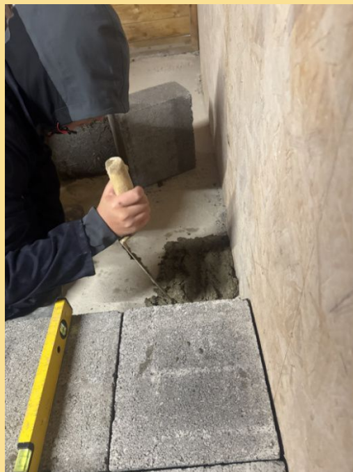
Cain student Dylan has been enjoying working in the construction shed with Alan. They are working on creating a fireplace!
